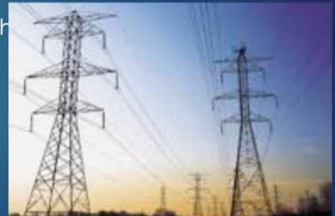
Power Grid Line
